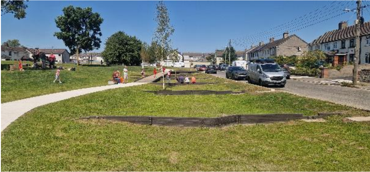
Retrofit SuDS – Swale in existing public open space, storing surface runoff and slowing the peak flow.
